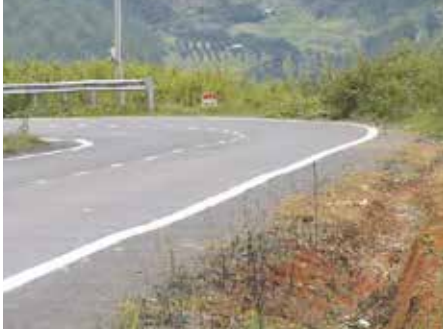
INSUFFICIENT PASSIVE SAFETY INSTALLATION: - OPEN WINDOW - END TREATMENT - KM- STONE IS AN UNPROTECTED OBSTACLE
