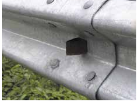
INSUFFICIENT PASSIVE SAFETY INSTALLATION: - REFLECTOR IS RUSTY AND OUT OF FUNCTION
