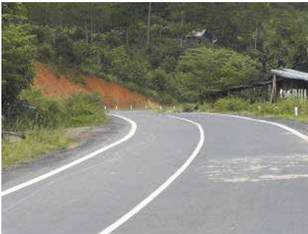
OBSTRUCTED VISIBILITY ON THE COURSE OF THE ROAD
