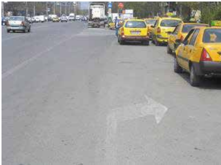
LINE MARKING IS NOT APPROPRIATE TO THE SITUATION AT INTERSECTION WITH SECUIOR, TAXI PARKING DISTRACTS ORIENTATION
