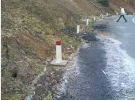
INSUFFICIENT ROAD DRAINAGE
