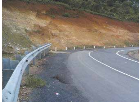
INSUFFICIENT PREVENTION AGAINST SLOPE EROSION AND LAND SLIDES AT KM229+060 –
