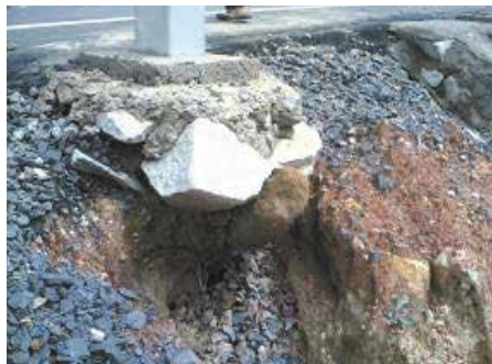
INSUFFICIENT FOUNDATION OF CRASH BARRIERS
