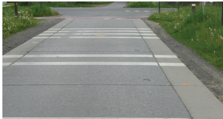
Illustration 53: Example of advanced visual cues of approaching intersections by use of optical break in Belgium [37]
