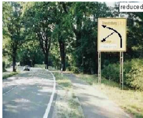
Illustration 73: Corrected direction of the sign is compatible with the road course and marking old course is concealed. [12]
